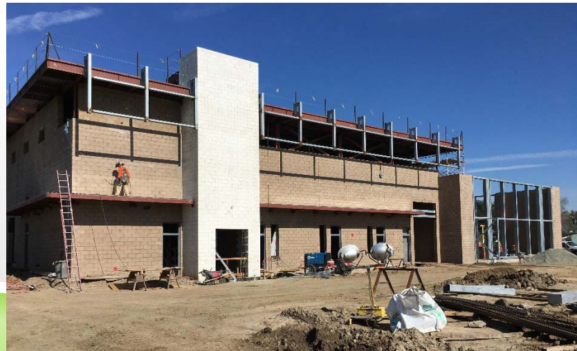
New Central Plant
